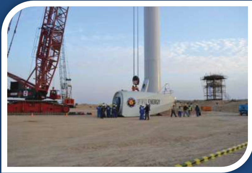
Nacelle on Ground
