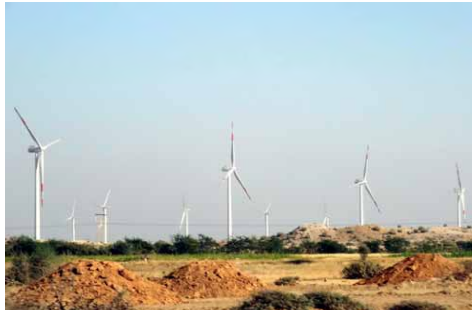
Zorlu Enerji Wind Power Project
